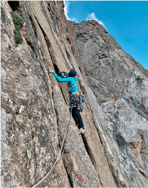
Federica Mingolla drilling a bolt placement during the establishment of Vivere la Vita on Wall of Dykes.
